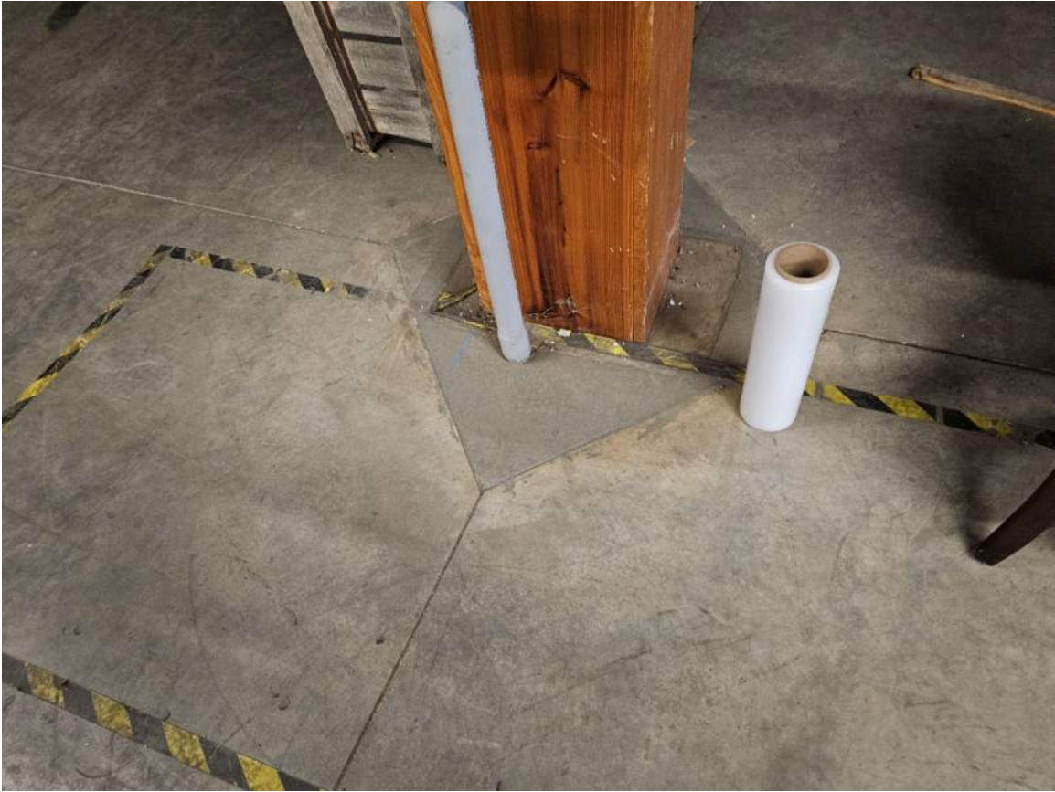
Photo #9 (Typical Interior Column Pedestal Condition – Building 1)
