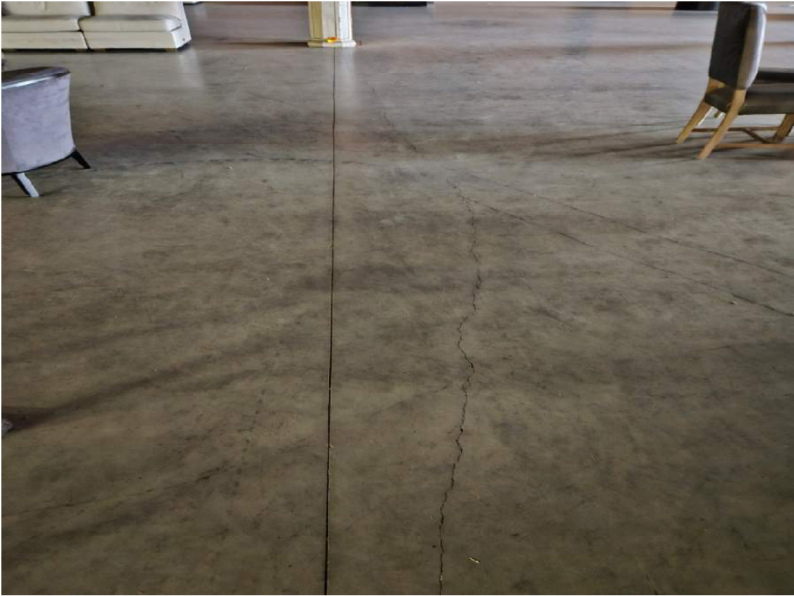
Photo #11 (Concrete Slab Cracking – Building 1)
