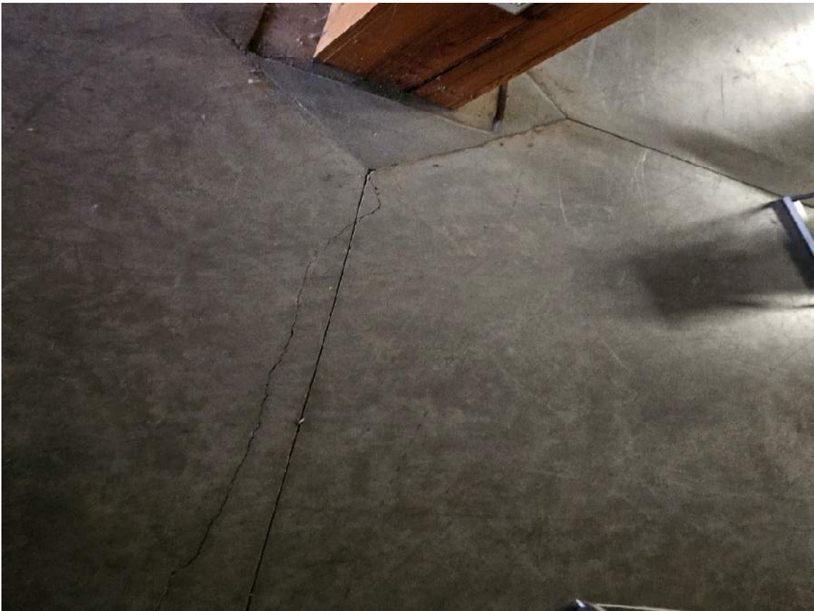
Photo #12 (Concrete Slab Cracking – Building 1)
