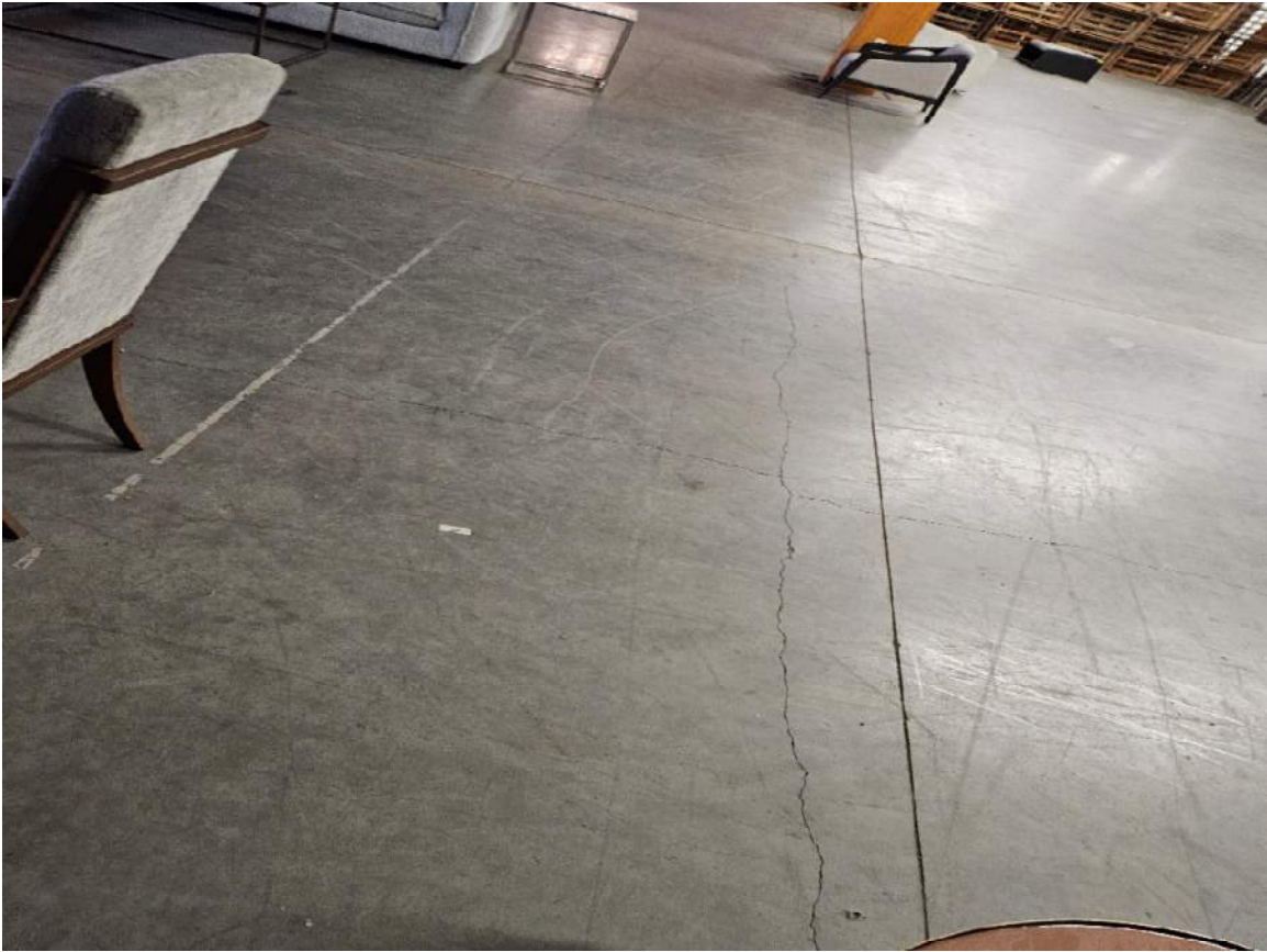
Photo #13 (Concrete Slab Cracking – Building 1)
