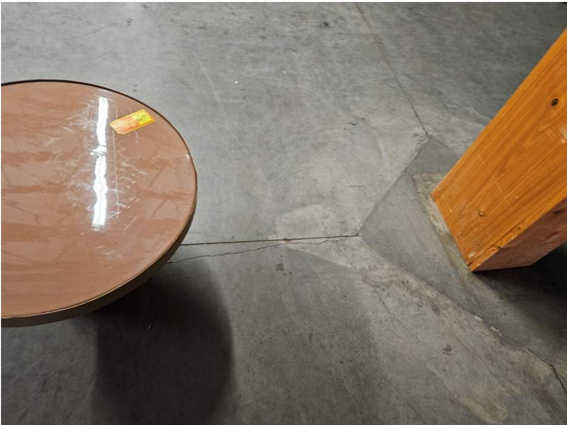
Photo #14 (Concrete Slab Cracking – Building 1)
