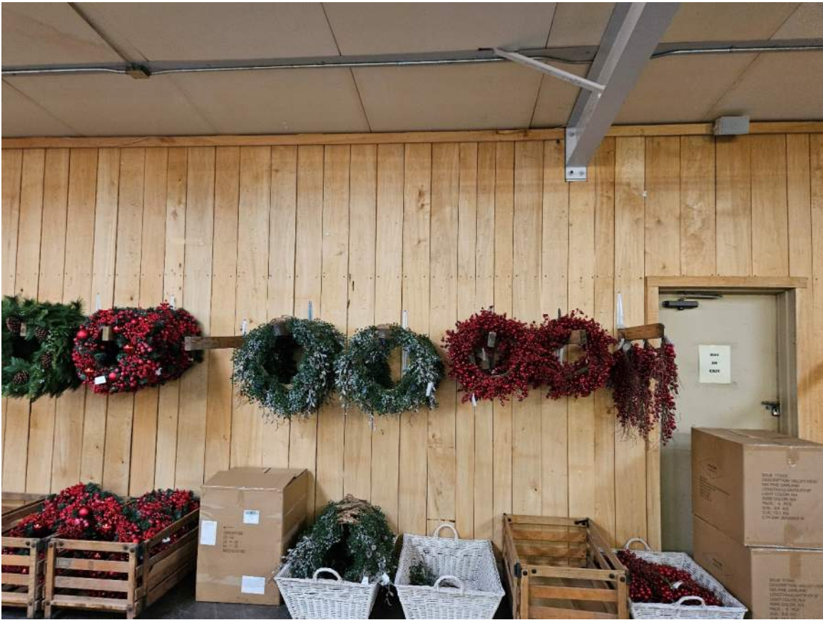
Photo #19 (Walls not exposed therefore couldn't see any bracing if present – Building 2)
