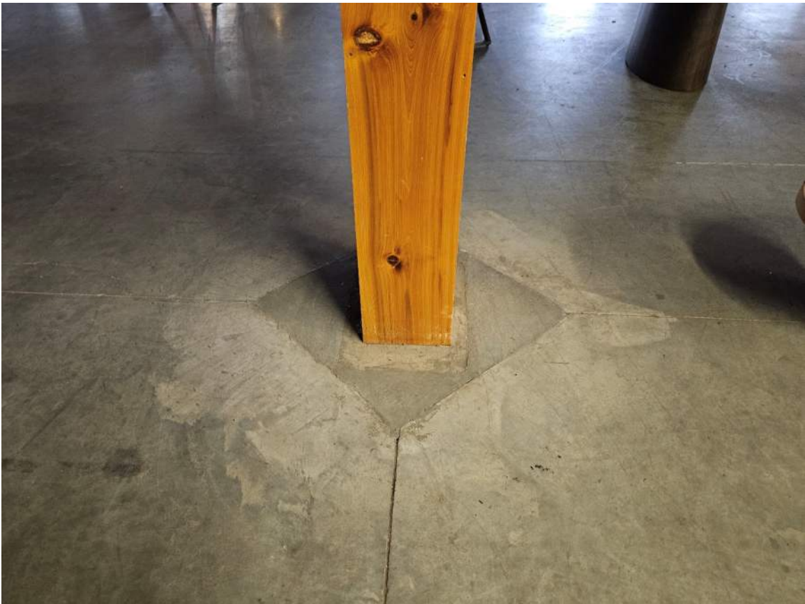
Photo #10 (Typical Interior Column Pedestal Condition – Building 1)
