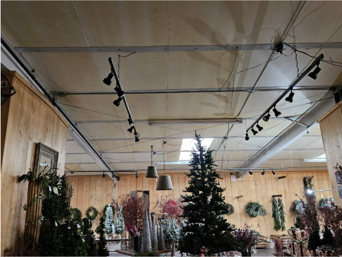
Photo #21 (Roof "X" bracing stops instead of continuing – Building 2)
