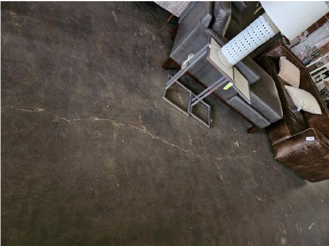
Photo #22 (Typical concrete slab cracking – Building 2)
